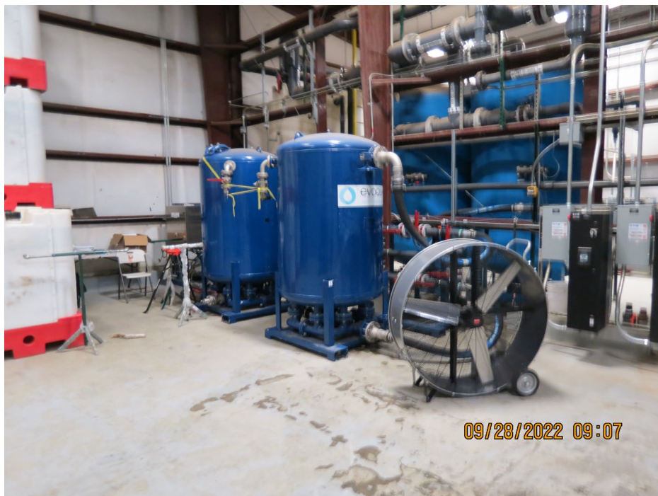
Figure 6. SEPTS New Perchlorate treatment units.
