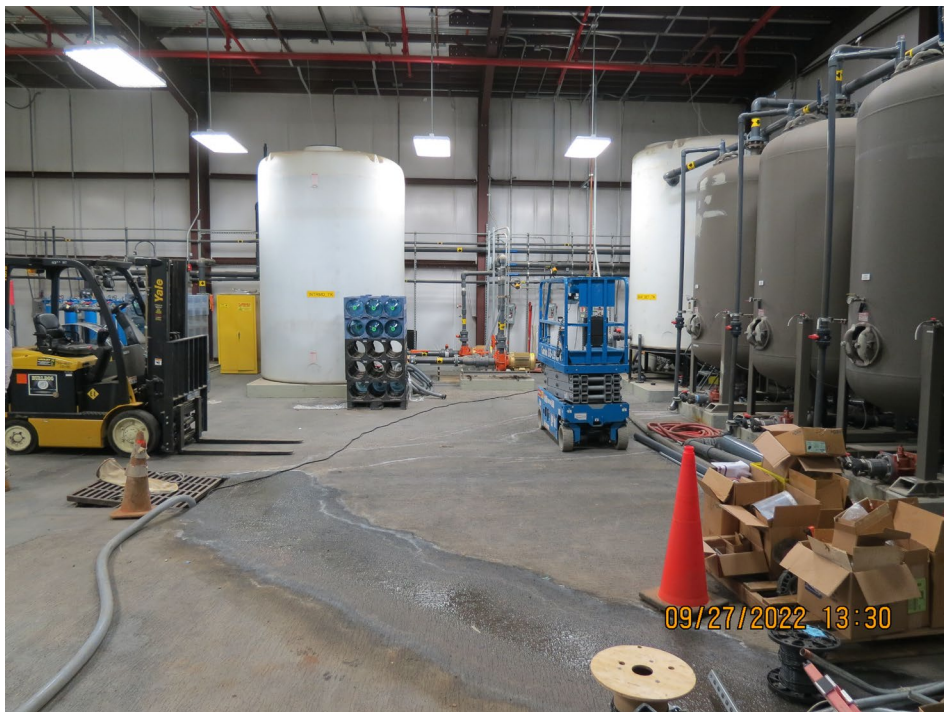
Figure 1. Playa 1 (P1PTS) Treatment Building, the system was inactive at the time of the Site Inspection and was undergoing modification to connect the new Pivot Irrigation System. Intermediate holding tank (center), GAC units (right side).
