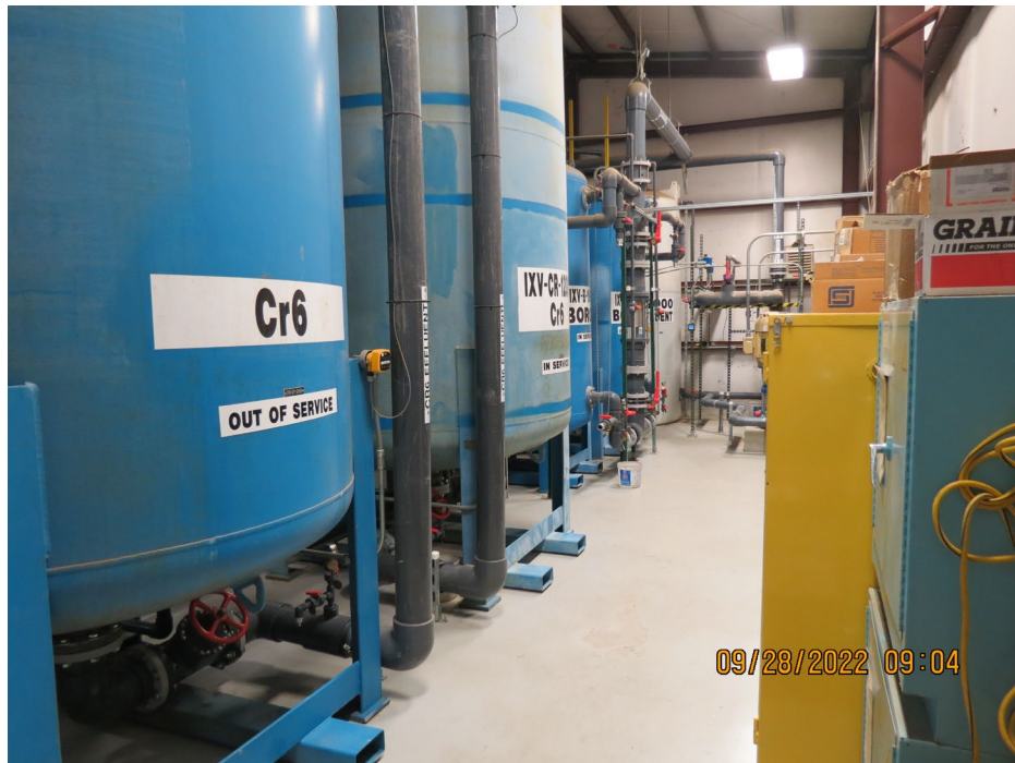
Figure 5. SEPTS Chromium and Boron treatment units.
