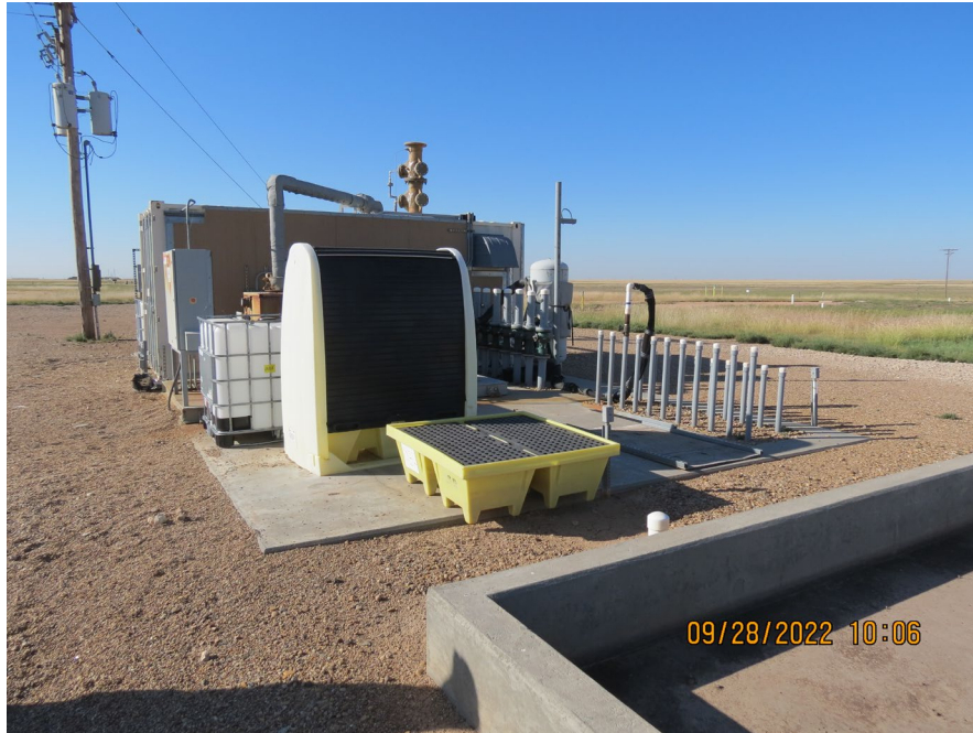
Figure 12. Burning Ground SVE System – CatOx unit, Conex container, and scrubber stack in the background, hose connecting SVE-S020 to the blower (center right)
