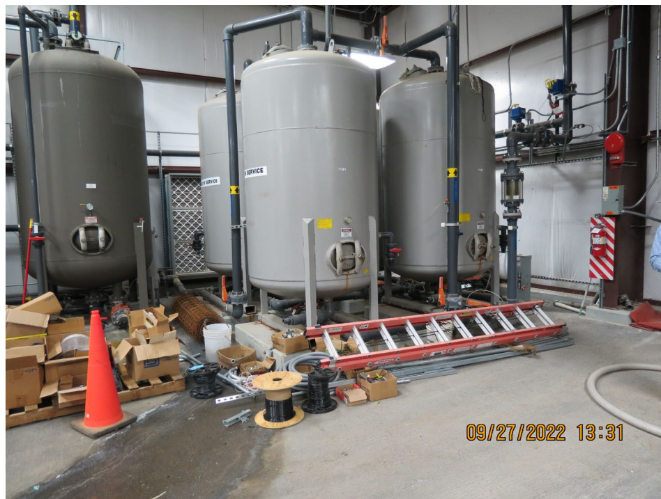
Figure 2. P1PTS four ion exchange units (right side), GAC unit (left side)
