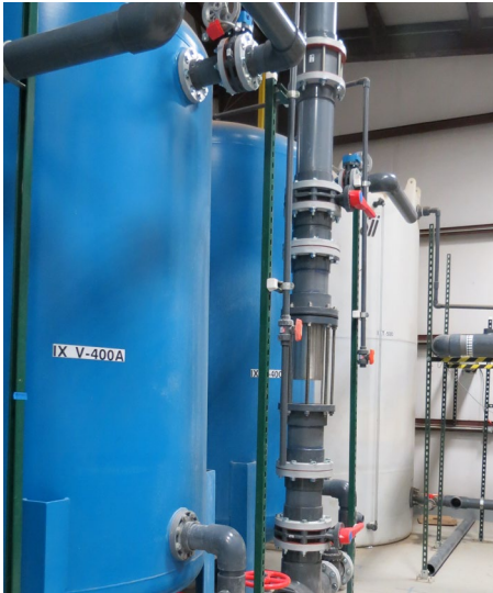
Ion Exchange and Effluent Tanks at SEPTS
